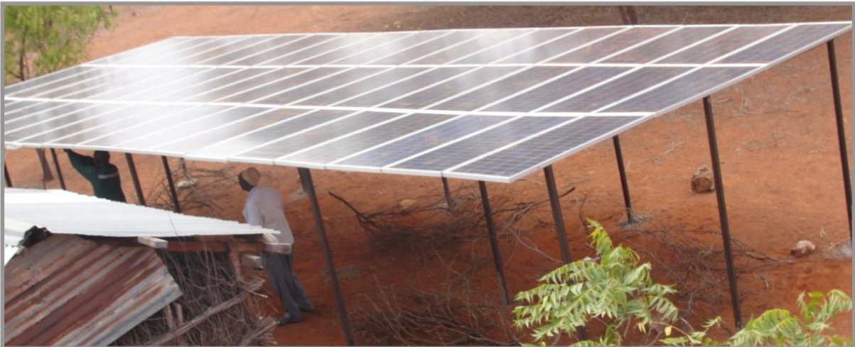
Complete Array of Solar Panels
